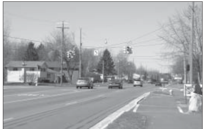
Using CDBG funds, Holland Charter Township expanded Riley Street to five lanes and improved its stormwater system.
